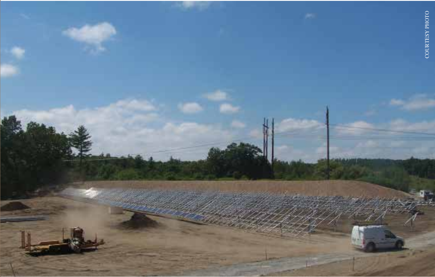
Construction is under way on Lancaster's solar array, which will be owned and operated by the town.
