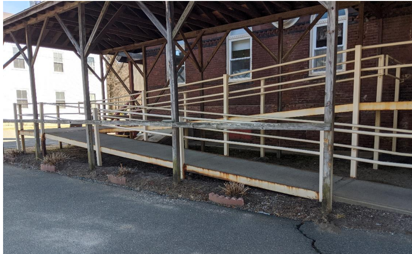
Photo of the rusting condition of the ramp at the Deerfield Regional Senior Center. Photo courtesy of the Town of Deerfield.
