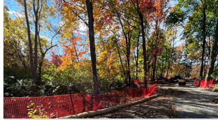
Reading has begun construction on a wetland water storage system in the Maillet, Sommes and Morgan conservation land. (Photo courtesy Horsley Witten Group)
