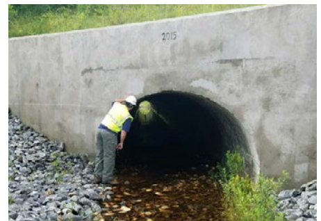
The Culvert Replacement Municipal Assistance Grant Program provides funding to remove or replace culverts in areas of high ecological value.
