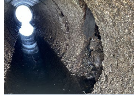
The interior of the culvert on Mattapoissett Neck Road shows evidence of deterioration. (Photo courtesy town of Mattapoissett)
