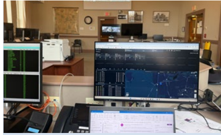
In its retrofit of the Town Council meeting room, Amherst added emergency dispatch equipment so that the room could also be used as an emergency operations center when needed. (Photo courtesy town of Amherst)
